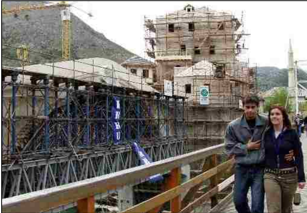
Figure 2.15: A temporary wooden bridge sits next to the Stari Most under reconstruction on April 9, 2004. Photograph from AP Photo/Hidajet Delic.
