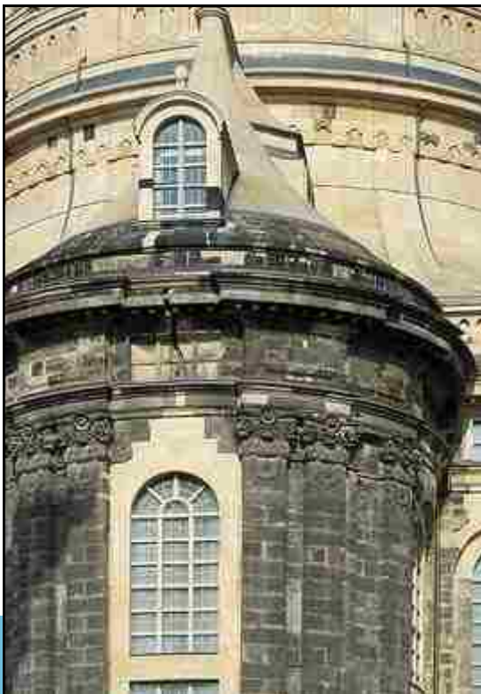
Figure 2.10: Detail of Frauenkirche reconstruction. The original material is distinguished from the new sandstone by staining. Photograph from Frauenkirche website. < www.frauenkirche-dresden.de >
